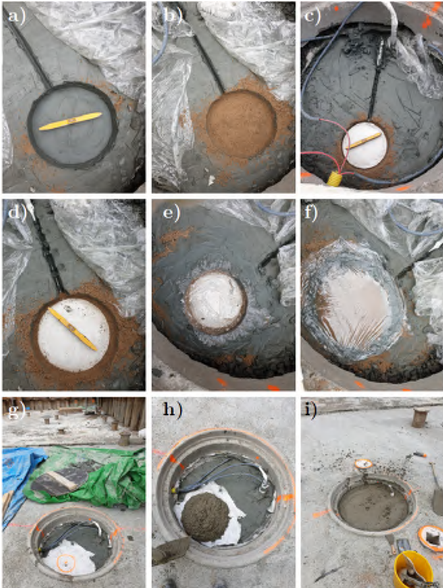
Figure C.23: Photos from installation of vertical earth pressure cells including final pouring of concrete over instruments.
